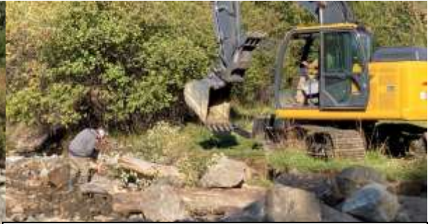
Figure 8. John Deere 130 Excavator at upstream extent of bank treatment showing placement of rootwads, logs and ballast rocks. Cottonwood and willow cuttings harvested from the site are being placed among the bank treatment.
