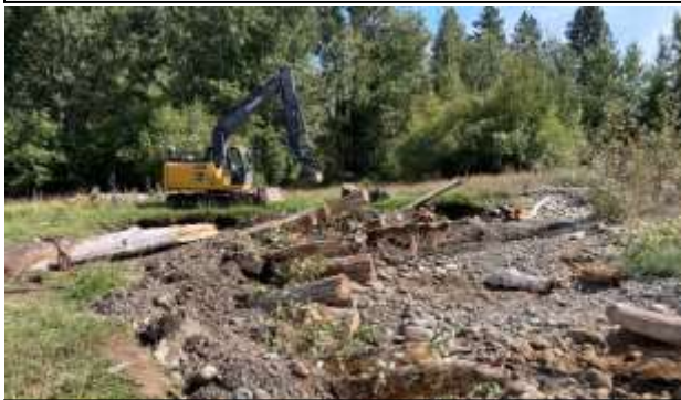
Figure 9. Close-up of willow and cottonwood cuttings placed within bank treatment after backfilling with channel sediment and trimming.
