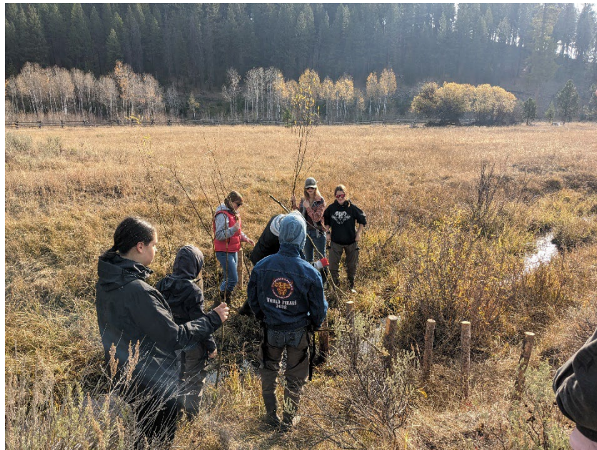
Figure 15: Baker and Unity high school students construct final BDA on Camp Creek.
